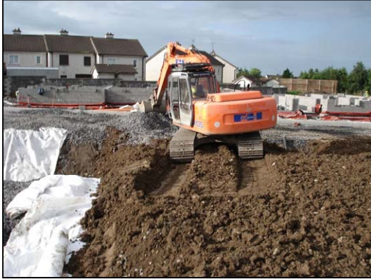
Fig. 13 – Track Machine Rutting
